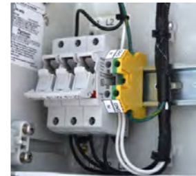
Fused voltage terminations
